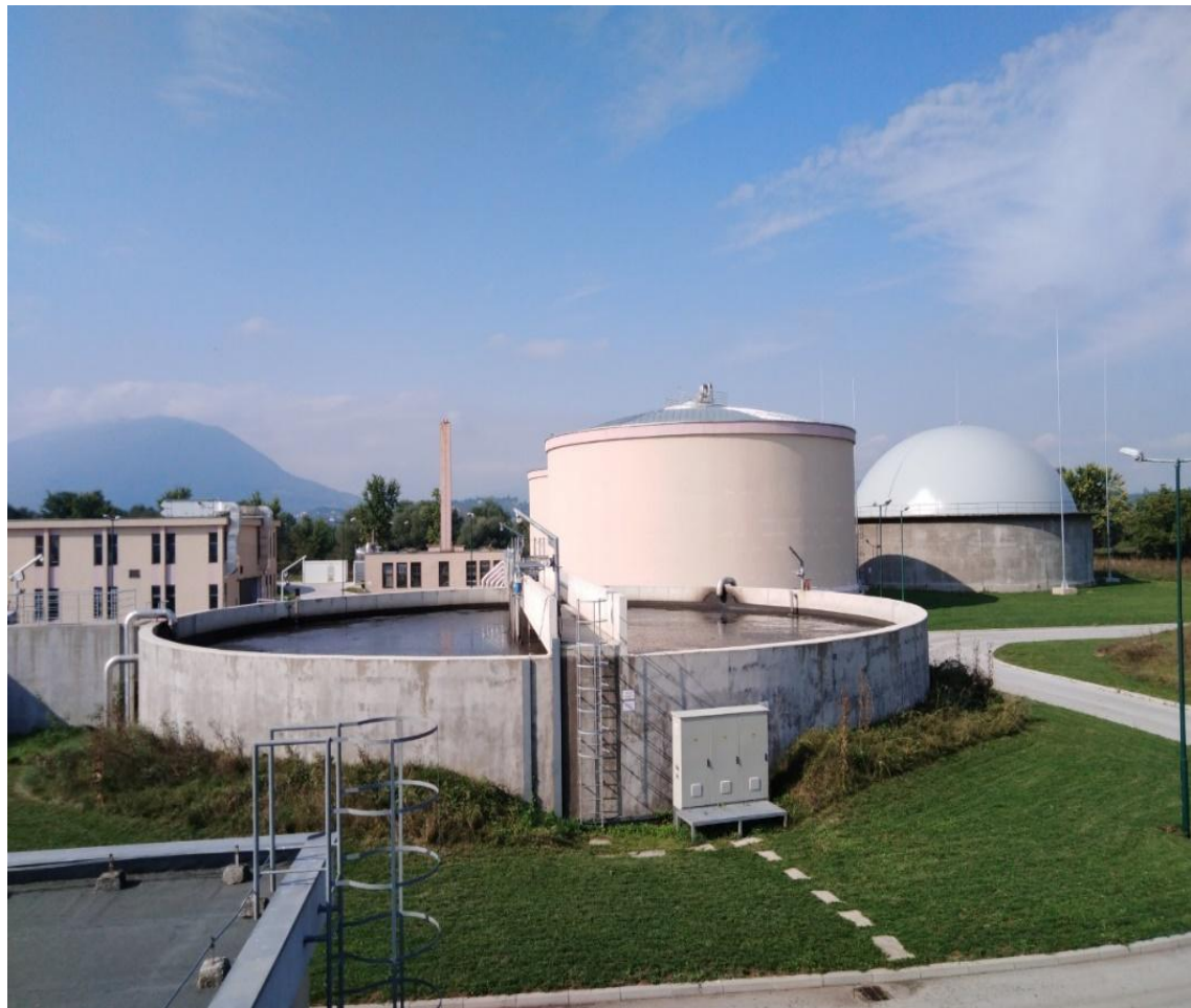
Mixed sludge tank, digesters and gas storage tank
