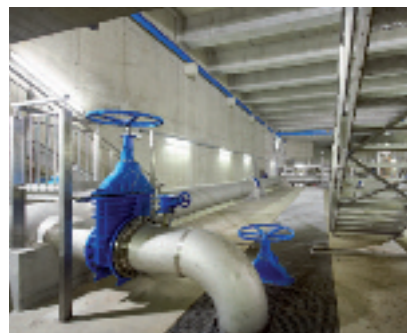
Pumping station, Wienerberg
