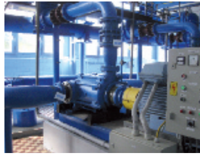
Tahi pumping station - Hungary
